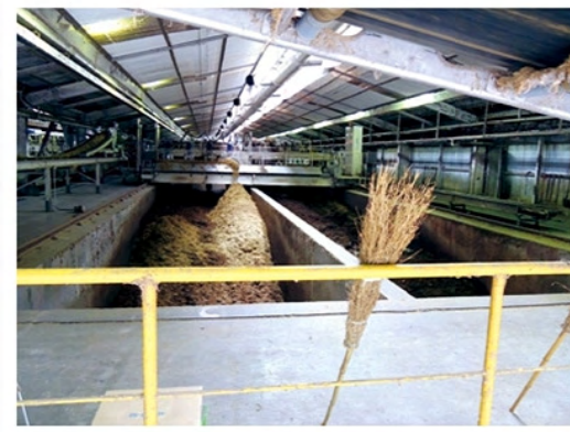
Waste management and recycling system 廢物處理及循環再造系統
